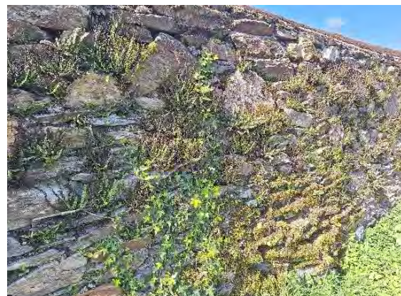
Profuse growth of mosses and ferns on the southern boundary wall
